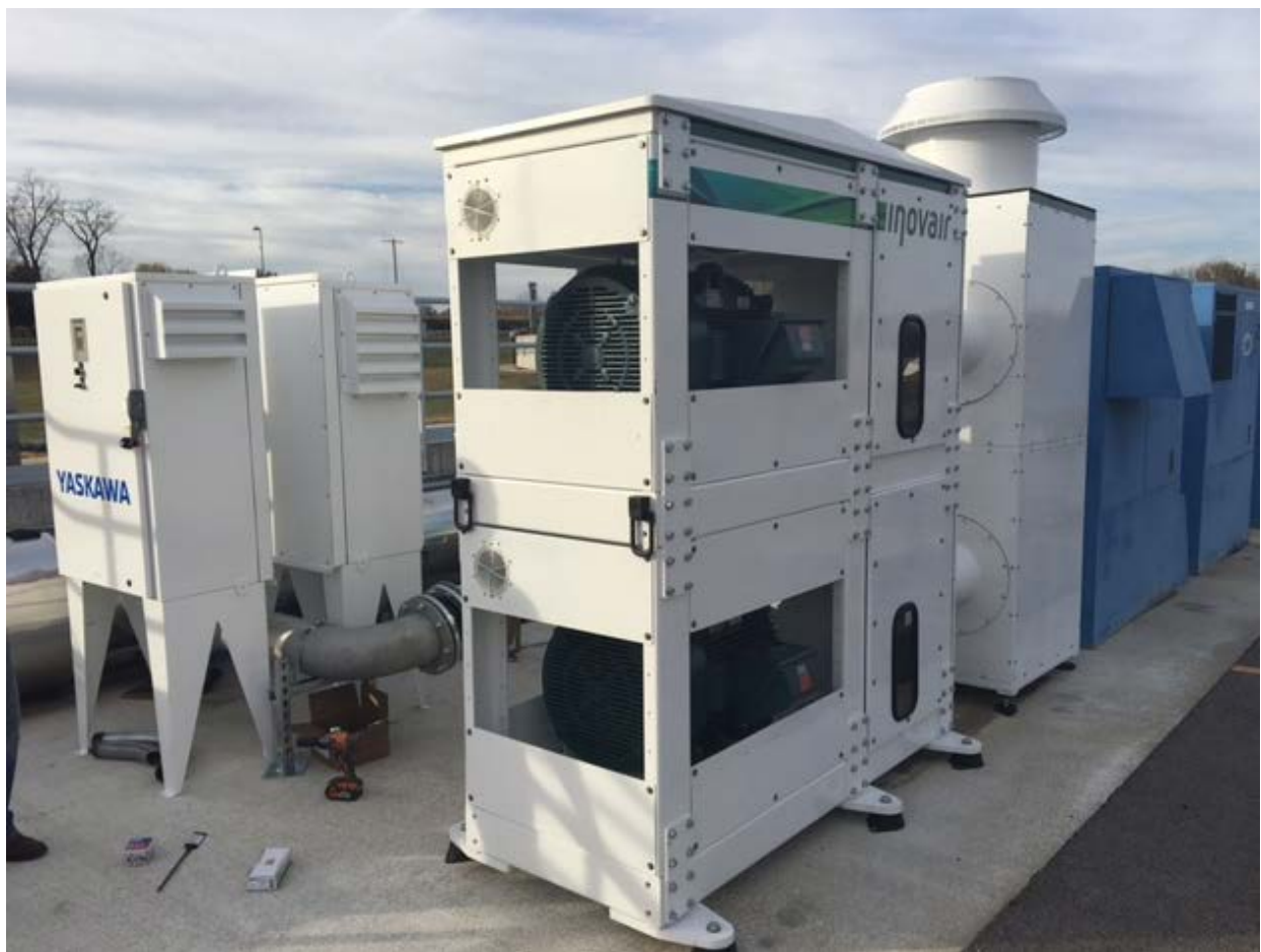
Figure 4: Prototype Inovair IM stack during installation, customer specified Variable Frequency Drives are visible in this outdoor installation.
