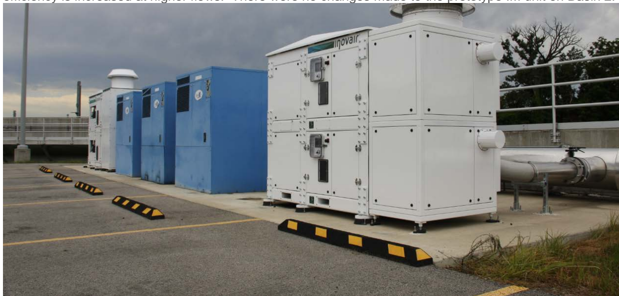
Figure 10: Inovair integrally geared centrifugal blowers installed alongside rotary lobe blowers. Production IM is nearest, prototype IM is visible in the background, 3 remaining rotary lobe blowers visible in the middle are unused, but fulfil the need for a redundant unit. There were initially 5 rotary lobe blowers, 2 per basin with 1 shared redundant unit. The Inovair Modular integrally geared centrifugal blowers physically replaced 2 rotary lobe blowers while functionally replacing 4 of them.
