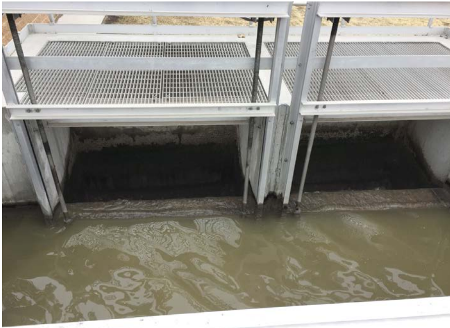
Figure 3: Product flow division between Basin 2 and Basin 3 at the Headworks Building
